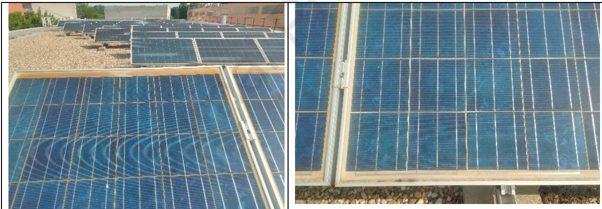
431 Figure 10.- Perspective image of the experimental and commercial areas with c-Si panels of the same model.
