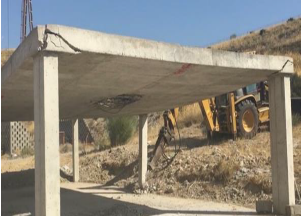
Figure 2.32: Cracks close to the end of the second central column removal.
