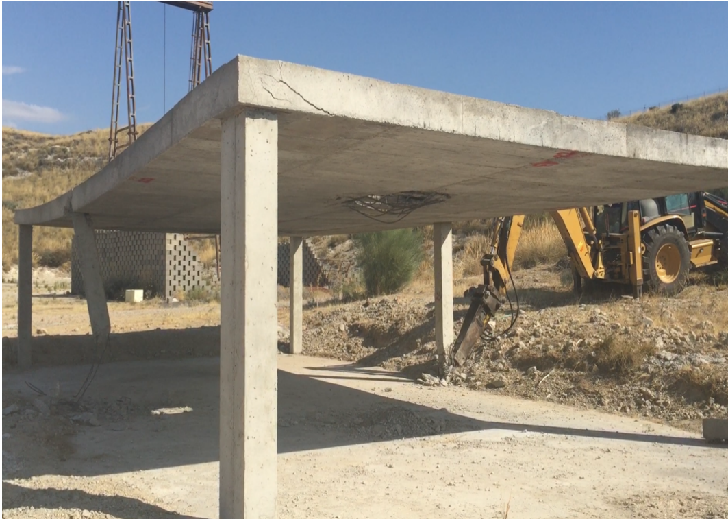
Figure 2.31: Cracks after one of the central supports was demolished.
