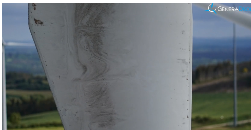
Figure 7.7: Image of a windmill blade obtained during the inspection. All rights reserved by Generadron S.L. 3
