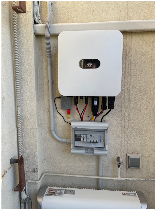
Figure 41. Installation in a real environment.
