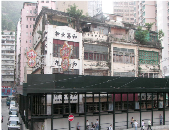
Fig. 161. Cluster of Tong Lau houses on Johnson Road before restoration. Source: author, 2008.
