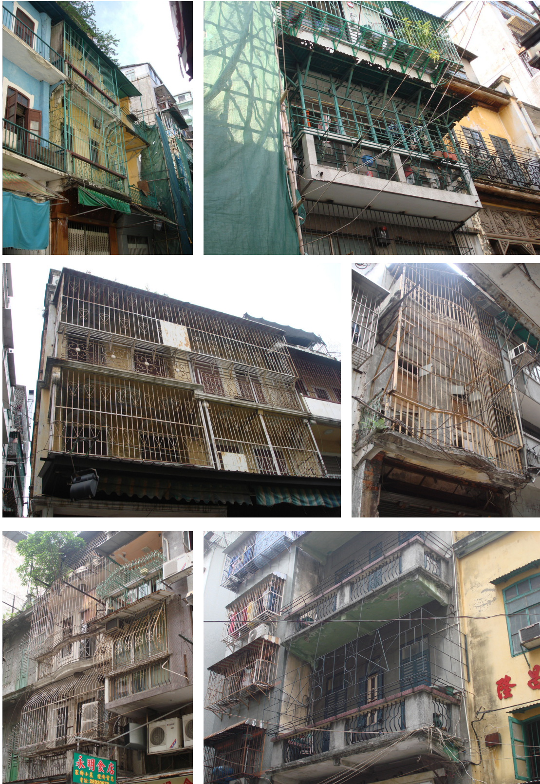
Fig. 168. Examples of non-compliant enclosures of balconies in old buildings (most of them built pre-war) in the Macau Peninsula. Some of them form structures of remarkable aesthetic value. Source: author, 2008.
