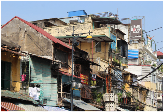
Fig. 310. Current state of the Sino-Vientamite houses in the Thirty-Six Streets Quarter, Hanoi, 2016. Source: author.
