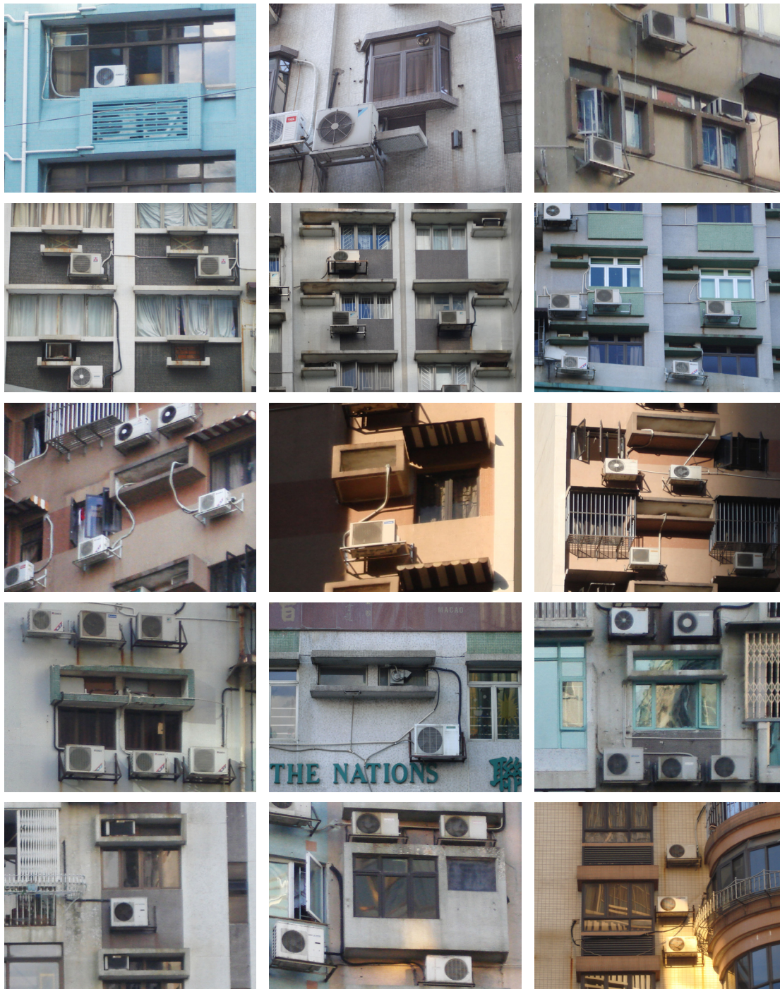
Fig. 367. Examples of maladaptations of air-con units to built-in façade receptacles in apartment buildings in Macau, 2008. Source: author.
