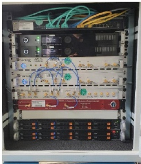
Figure 5.13: Rack of SABBIA 2.0 passive radar system including the front-ends, reference signal synthesizer, controlling units and recording computers.
