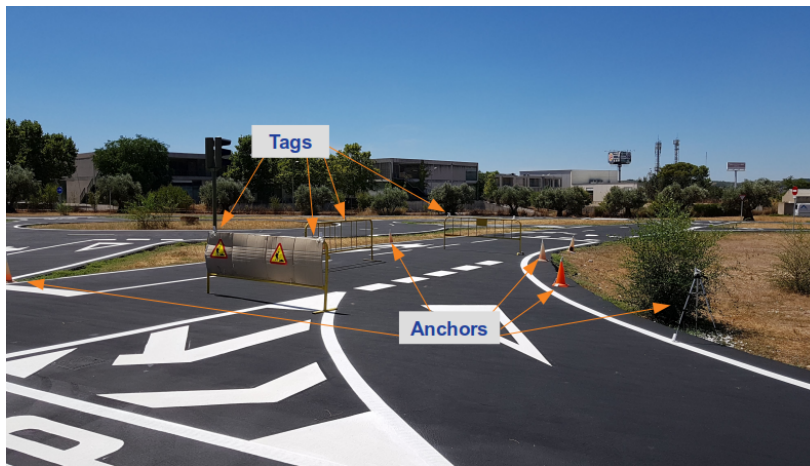
Figure A.4: Example of roadworks area reported through V2X communications [41]. The area covered by the roadworks is delimited by fences and estimated using Ultra-wideband (UWB) sensors installed on the road infrastructures.
