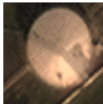
(k) Storage tank
