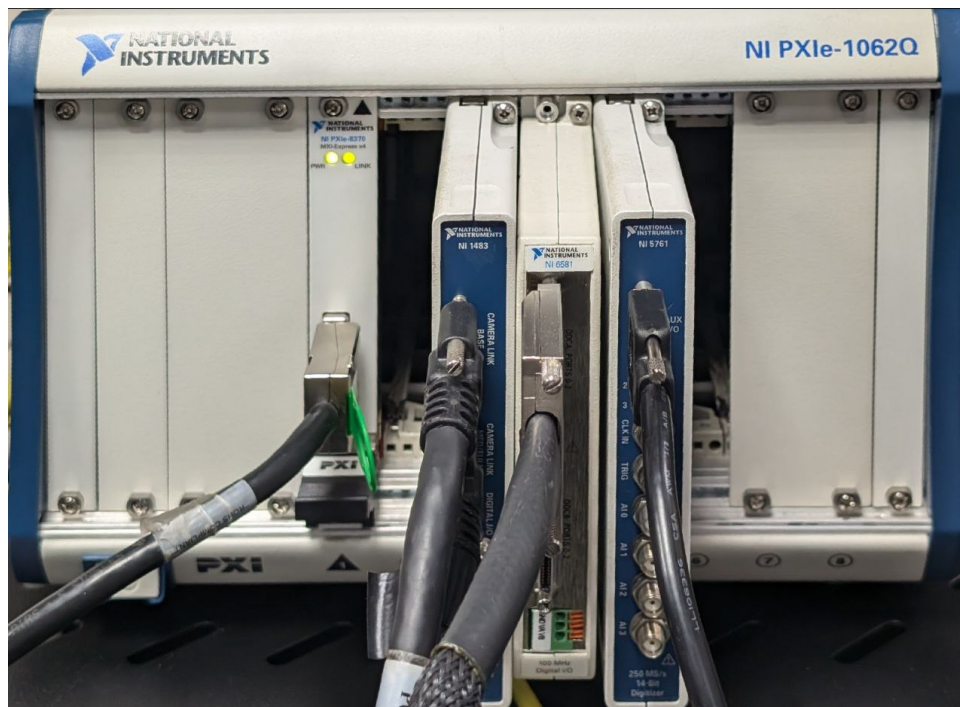
Figure 3.28: Chassis with the FlexRIO boards used during development
