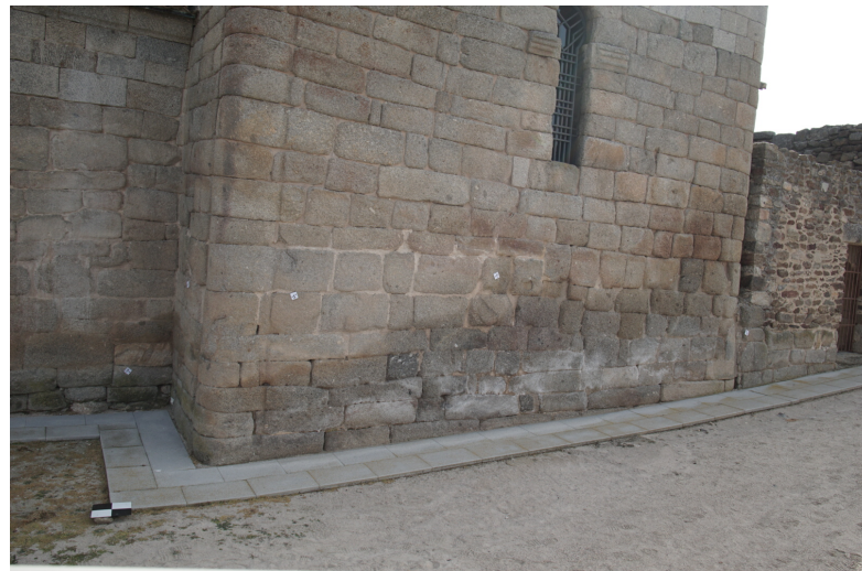
Figure 21. Pathology in north façade of the building.
