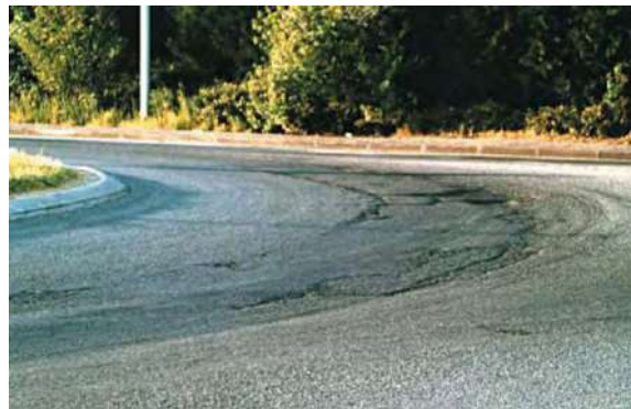
Figure 2.46: Deformation and loosening of aggregates due to the effects of the tangential forces of the tires. Source: (Hamlat et al., 2007).
