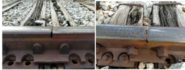
FIGURE 20 Rail with flange joint without welding, confirmed during visual inspection.
