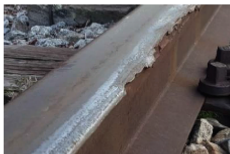
FIGURE 29 Surface defects on railway rails.
