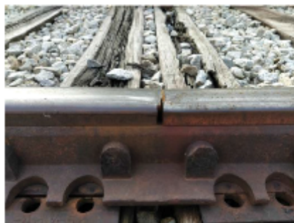
FIGURE 28 Poor condition of junctions with flange joint.
