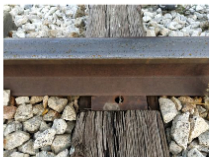
FIGURE 30 Lack of bolts.
