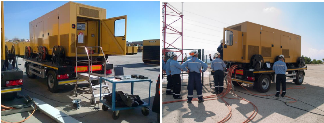
Figure 3.5: Portable diesel generator FLEX-DG for use in FLEX strategies [ANAV, 2013]
