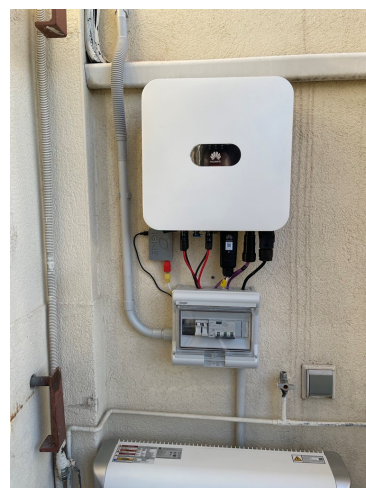
Figure 29. Installation in a real environment.
