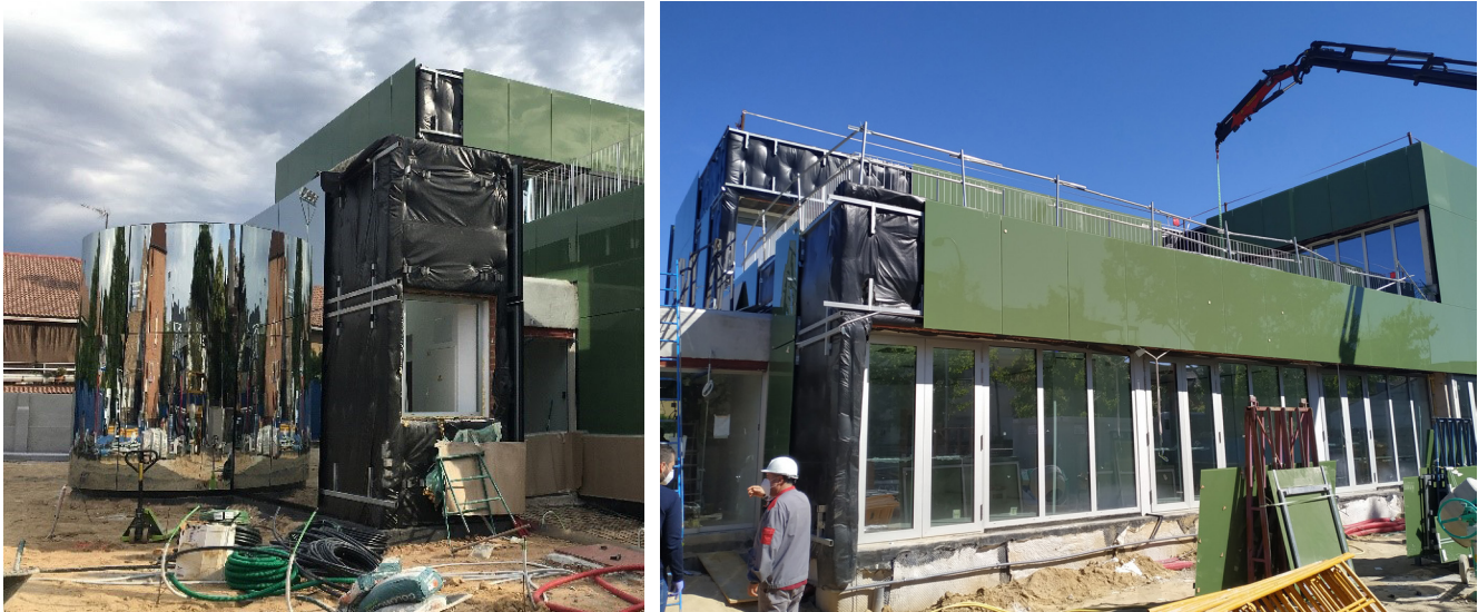
Figures 14. Construction of the BRAINS school. Placement of curved mirrors and glass in the envelope.
