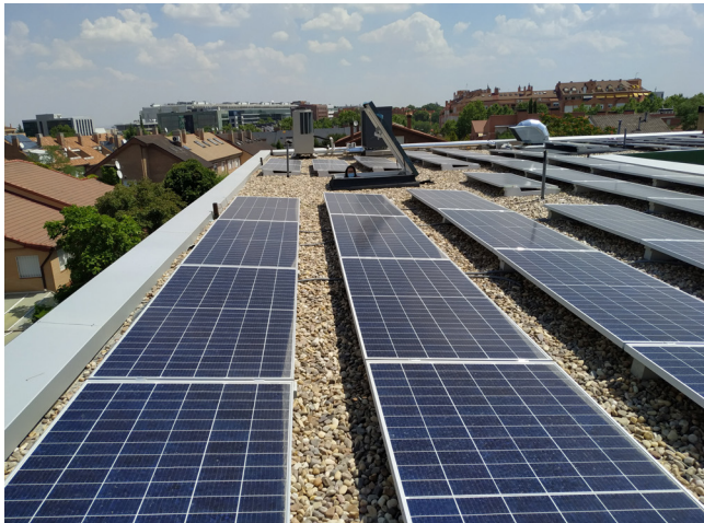
Figure 3. Photovoltaic solar panels on the rooftop.
