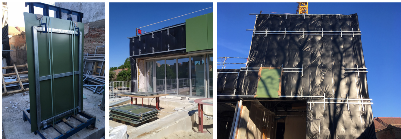
Figures 2. Large thicknesses of continuous thermal insulation throughout the building skin. Carpentry with tripalut glass.
