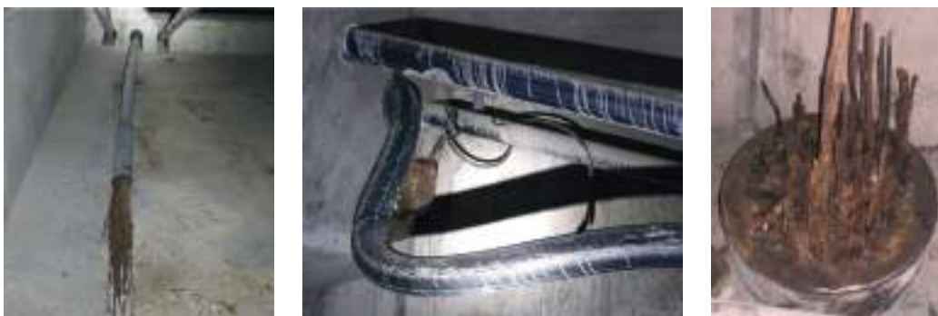
Figure 2: Broken tendon affected by corrosion [1].
