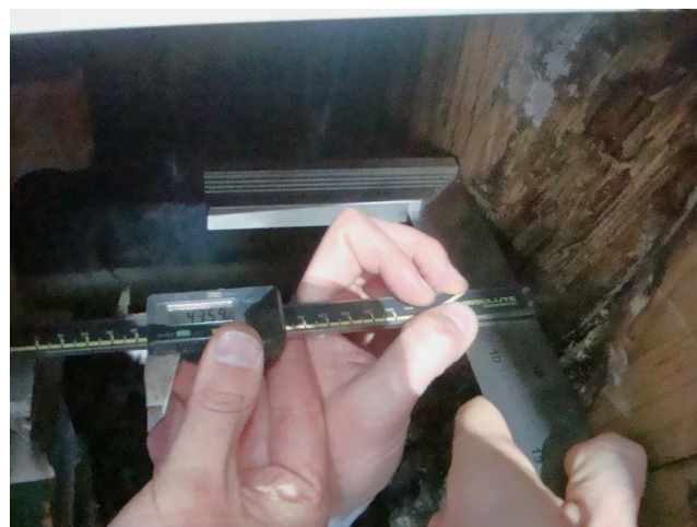
Figure 7. Measurement of sectional loss due to wood rot using a digital caliper.
