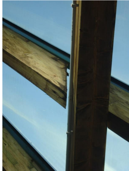
Figure 9. Breakage of fixings between the pair and beam.
