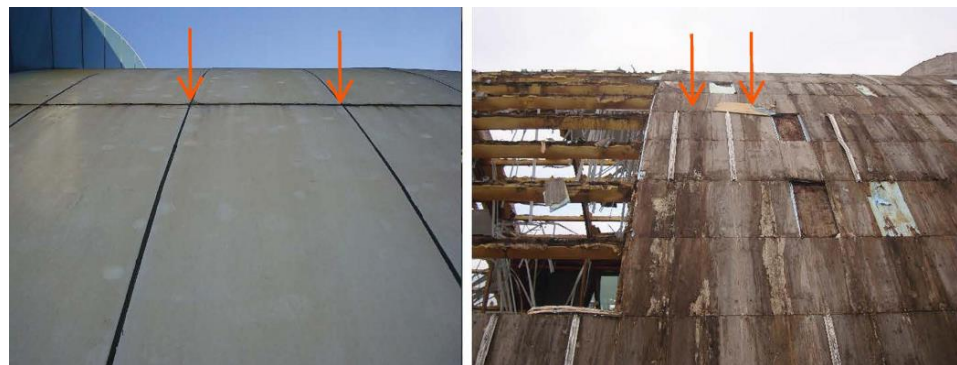
Figure 16. Left of the image: composite roof panels before demolition. Right of the image: the wooden sandwich panel during the demolition process. Red arrows indicate areas of water seepage through the composite roof panels.
