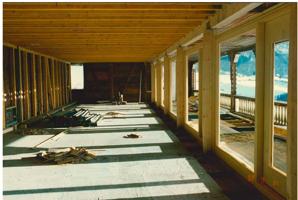
Figure 8. Walenstadtberg Housing. Timber frame construction on the second floor. Note the southwest façade featuring a glazed loggia and the entasis of the three pillars to the right. Material provided by Gody Kühnis.
