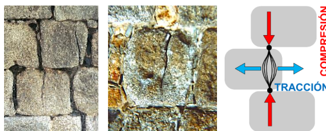
[44] Salamanca. Puente Mayor, sillares rotos [45] causa
