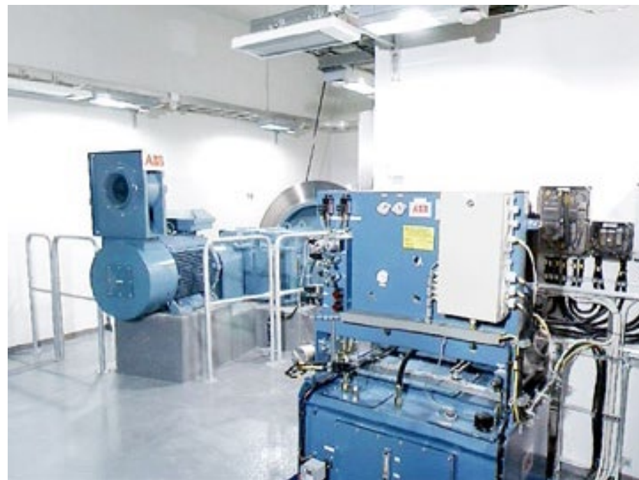
Single drum hoist (Source: ABB)
