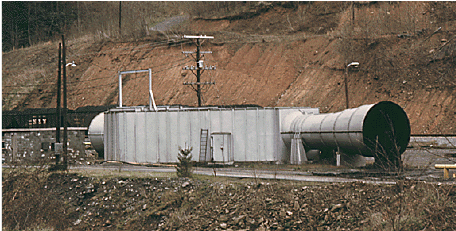
Large fan equipment used to blow fresh air into Virginia-Pocahontas Coal Company mine #2 near Richlands, Virginia. Fuente: Environmental Protection Agency.
