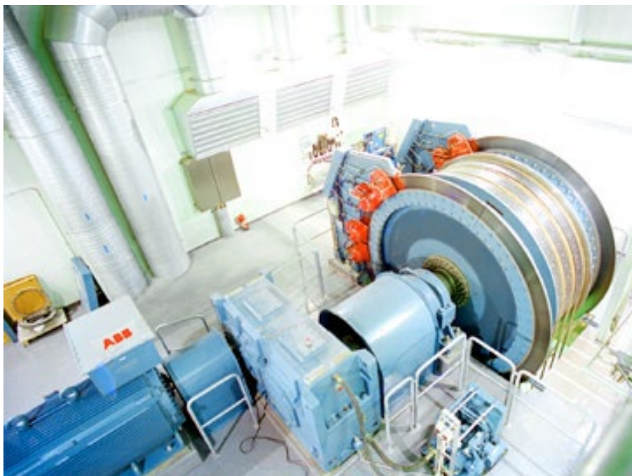
Tower mounted friction hoist with low voltage motor (Source: ABB)
