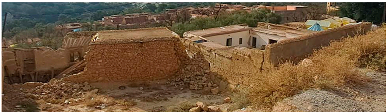
Figure 12. Impact of the 8 September 2023 earthquake on a traditional building in Adassil with a floor made of wood, straw, and mud. The observed damage includes the disintegration of sections of the stone masonry walls of the house and failure characterized by perpendicular bending at the corners of the rammed-earth dwelling.
