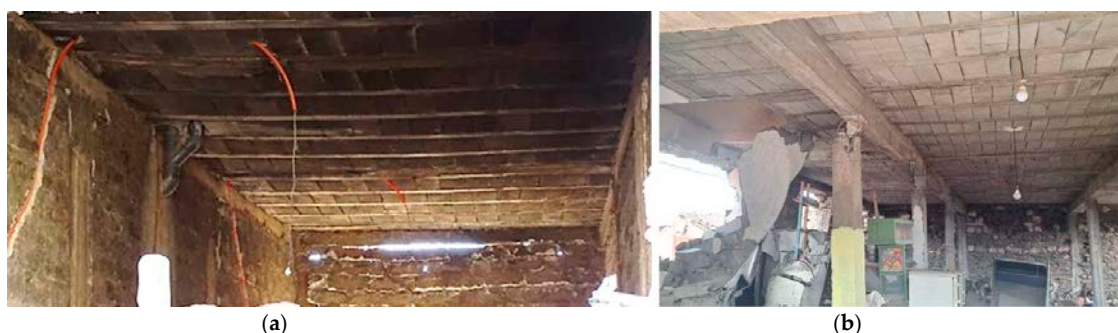
Figure 26. Buildings presenting a structural system which provides seismic resistance and stiffness mainly in only one of the two orthogonal directions. (a) Amizmiz; (b) Tafeghaghte.
