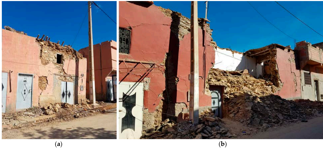
Figure 11. Impact of the 8 September 2023 earthquake on a stone masonry building with wooden log slab in Amizmiz. Image (a) illustrates the inward collapse of the roof, attributed to inadequate support, leading to the subsequent collapse of the upper part of the wall. Image (b) shows the crumbling of the walls.
