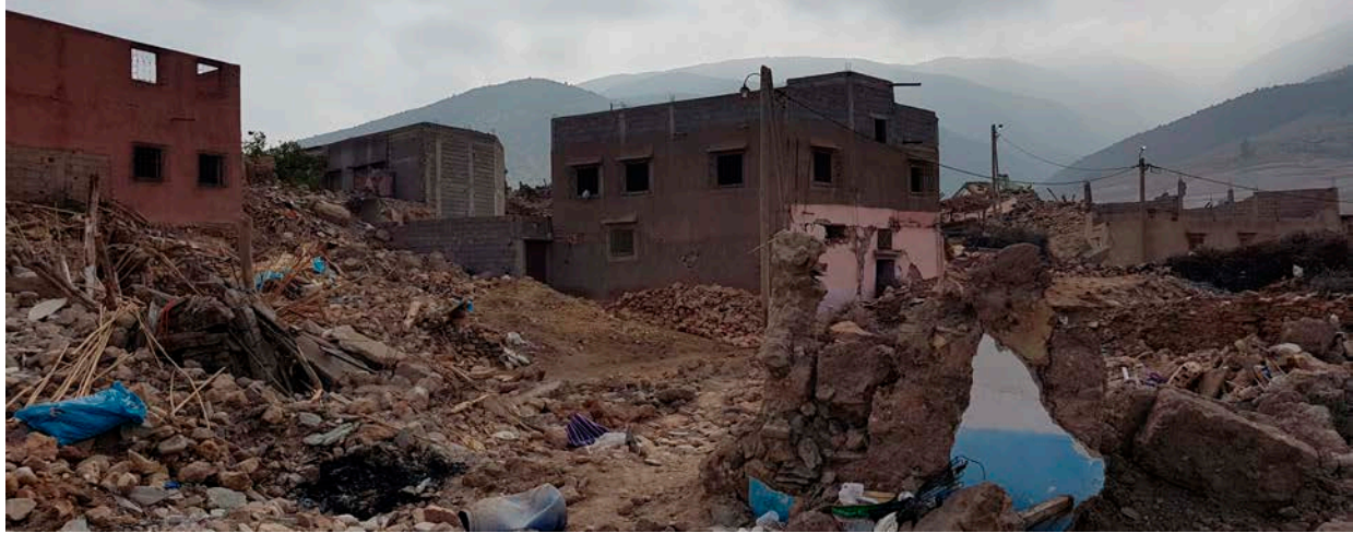
Figure 7. Evaluation of damage along a street in Tafeghaghte subsequent to the 8 September 2023 earthquake. Stone masonry structures have predominantly collapsed, while confined masonry systems or confined mixed systems mostly display damage ranging from grade 2 to 4 [31].
