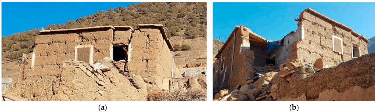
Figure 13. Damage assessment of a traditional rammed-earth building depicting various stages of damage. The corner failure is exacerbated by the presence of window openings. (a) Partial corner failure, (b) Total corner failure.
