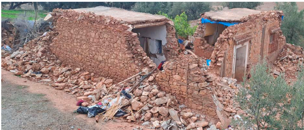
Figure 14. Damage observed in an L-shaped masonry residential structure. The damage at the corner is evident, attributed to concentration of stress in this specific area. Residential dwelling in the vicinity of Tafeghaghate.
