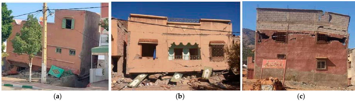
Figure 27. (a) Building in which the minor presence of shear-resistance walls on the ground floor resulted in a weak ground-story overturning failure (Amizmiz). (b) Building in which the excessive number of doors on the ground floor, which is characteristic of commercial buildings in the same road, causes a weak ground-story overturning failure (Talat N'Yaaqoud). (c) Building with major damage mainly concentrated in the intermediate story, due to window openings (Amizmiz).
