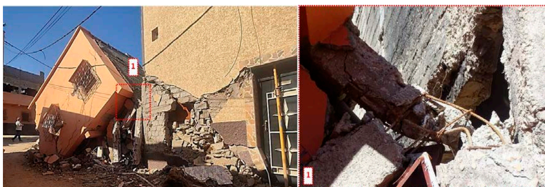
Figure 31. Building located on a corner, collapsed and overturned, presenting a possible weak-story deficiency and pounding effects from the adjacent building. Detail 1. Low resistance of the concrete and areas of low-longitudinal-reinforcement steel in the beam and the column. Short length of development and anchoring of steel for longitudinal reinforcement of the beam where it connects with the column. Absence in the beam of the recommended first closed confinement stirrup located no more than 50 mm from the face of the support element (ACI-318). Excessive distance between transversal reinforcement in a critical point of the column and absence of seismic hooks at the ends of the column stirrups (Amizmiz).
