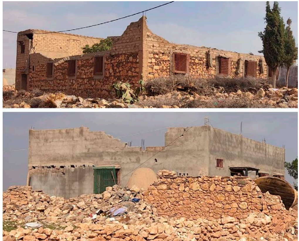
Figure 24. Out-of-plane failure of confined masonry parapet walls in two buildings with different structural wall material (Tafeghaghte) (both).
