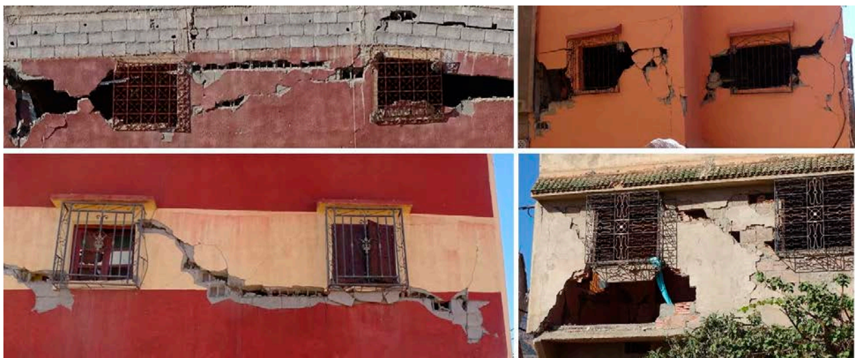
Figure 25. Damage mainly due to the absence of reinforced-concrete confining elements in door and window openings (Amizmiz) (all).
