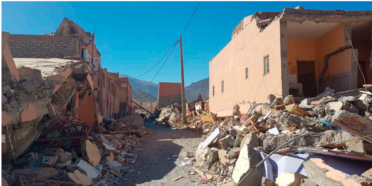
Figure 8. Assessment of damage in a street of Talat N'Yaaqoub following the 8 September 2023 earthquake. Confined masonry structures exhibit extensive destruction, with buildings suffering grade 3 or higher damage, and numerous collapses recorded at grade 5 [31].
