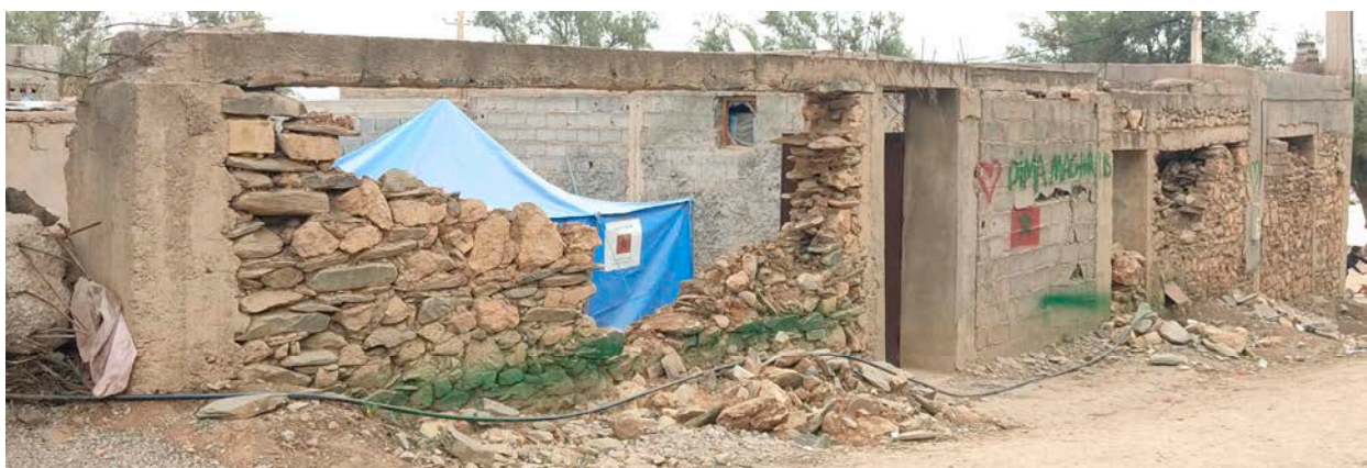
Figure 22. Comparison of damage for different infill materials in the same wall (Tafeghaghte).
