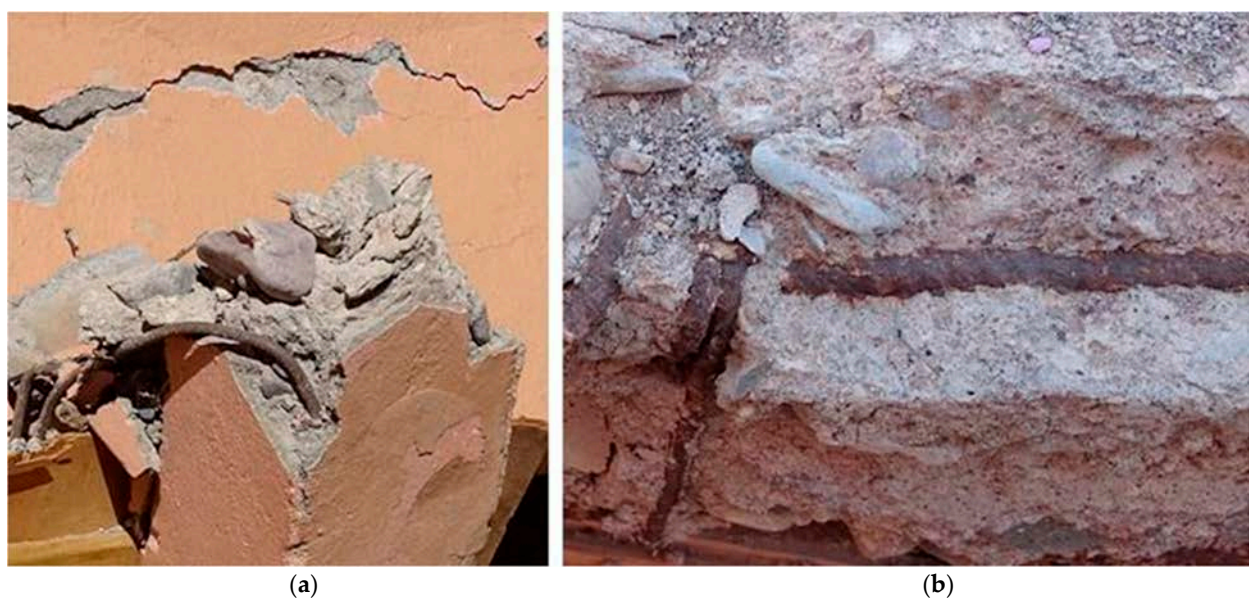
Figure 19. Deficiencies in steel bar reinforcement in concrete elements: (a) smooth bars; (b) presence of corrosion and minimal transversal ribs in longitudinal reinforcement (Talat N'Yaquod).
