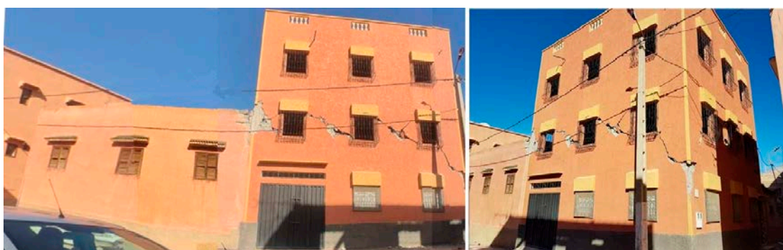
Figure 30. Building on a corner where a lower, more rigid adjacent construction has caused very noticeable pounding effects (Amizmiz).
