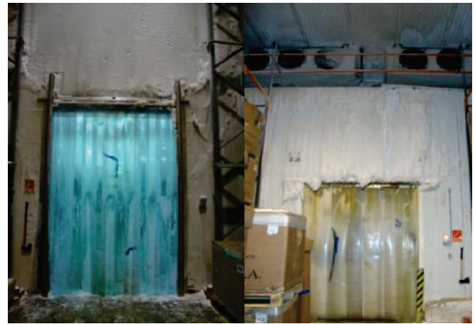
Fig. 2. Ice effect outdoors (left) and indoors (right) of the cold storage room.
