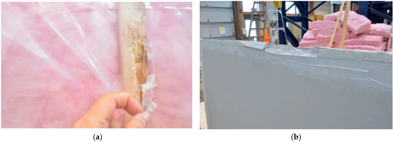
Figure 9. Material damage: (a) condition of the vapor barrier (polyethylene); (b) damage to the edge of the gypsum board.
