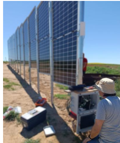
Figure 1: Agrivoltaic system with vertical bifacial PV panels
