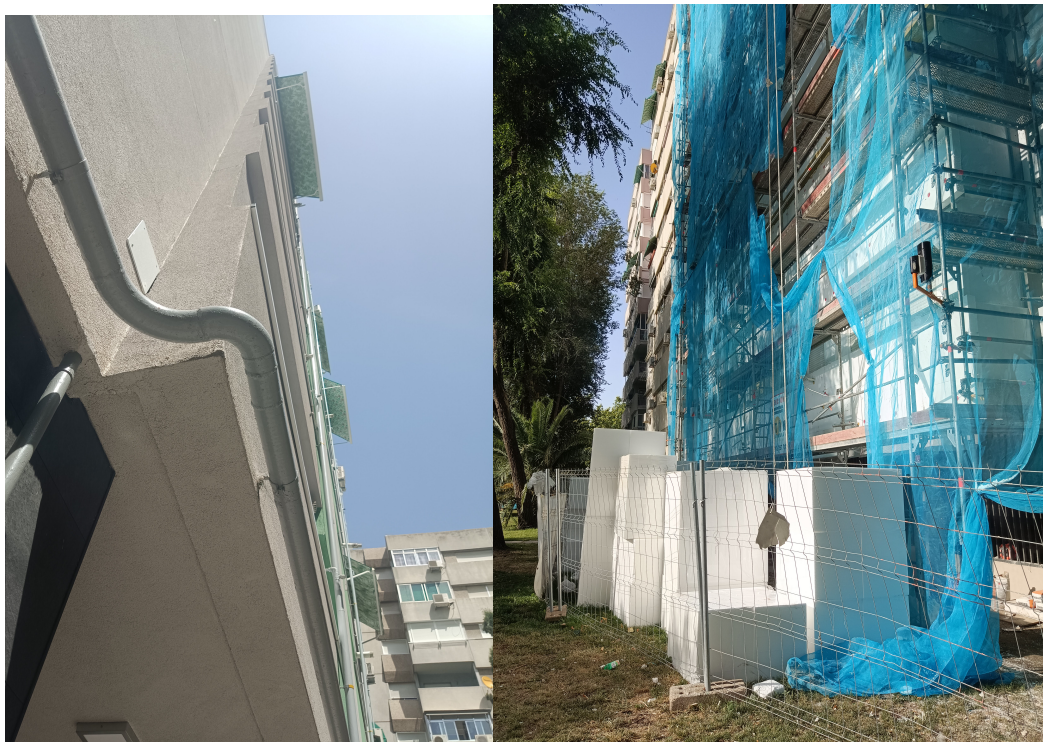
Figure 5.12: The SATE system (Exterior Thermal Insulation System) on a building under construction and another completed building in Poblado de Orcasitas
