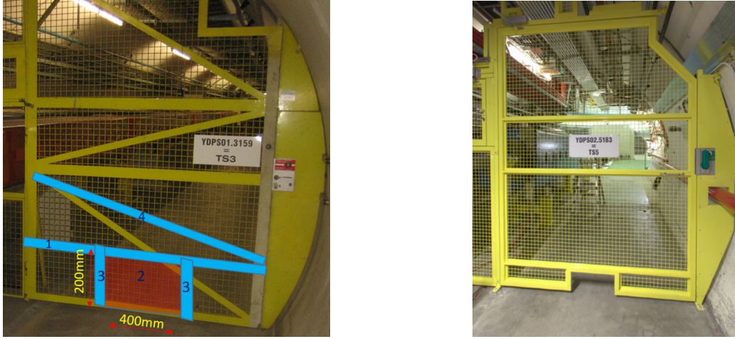
Figure 1.4: Safety gate modification for robot pass through.
