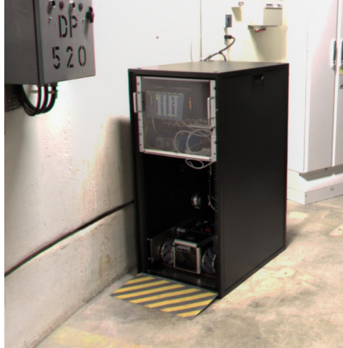
Figure 5.8: Charging station layout in the SPS tunnel.
