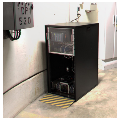
(b) Charging station installed in the SPS tunnel for automatic docking and recharging.
