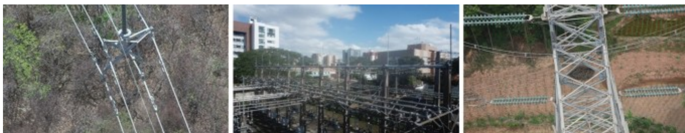
Figure 3. Representative samples from three evaluation datasets, highlighting the diversity of real-world object detection challenges. (Left) InsPLAD-det, showing power line infrastructure components with varying scales and complex backgrounds. (Middle) Electric Substation, featuring densely arranged objects and challenging lighting conditions. (Right) Bird’s Nest dataset, capturing aerial views of nesting sites on electrical towers. These datasets collectively represent the target scenarios for deploying resource-efficient YOLO models in critical infrastructure monitoring.
