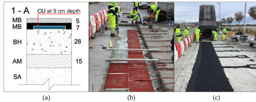
Figure 2. Experimental section from the CARDHIN project. (a) Typical pavement section 1-A. (b) Installation of the charging units (CUs). (c) Laying and compaction of the asphalt overlay.
