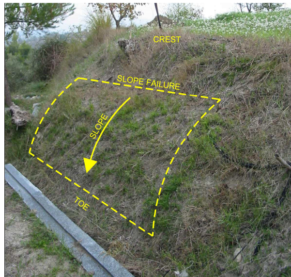
Figure 5 Observed slope failure at the study site (Mickovski and van Beek, 2009). Runoff over the slope contributed towards the loss of toe support, resulting in bulging mid-slope and deposition of soil material at the toe of the slope
