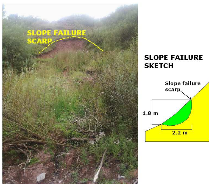
Figure 6 Slope failure in the study site
