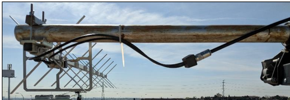
Figure 10. RF equipment connection to the communication antenna
